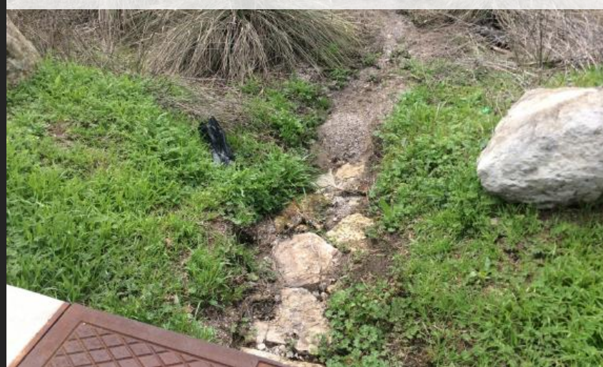
SCOURING AROUND INFLOW
