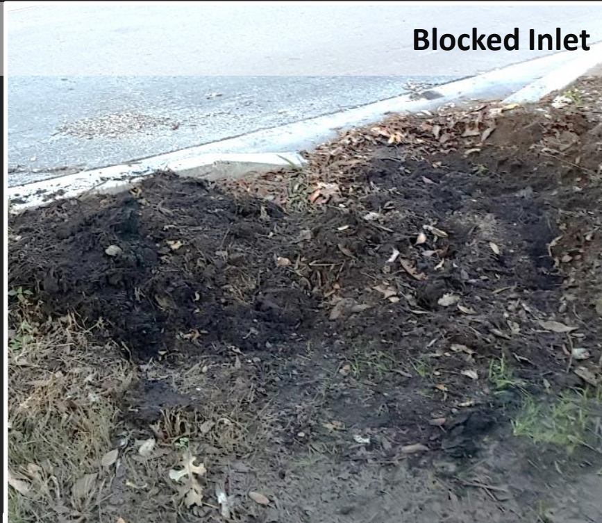
Basin Filled with Sediment
