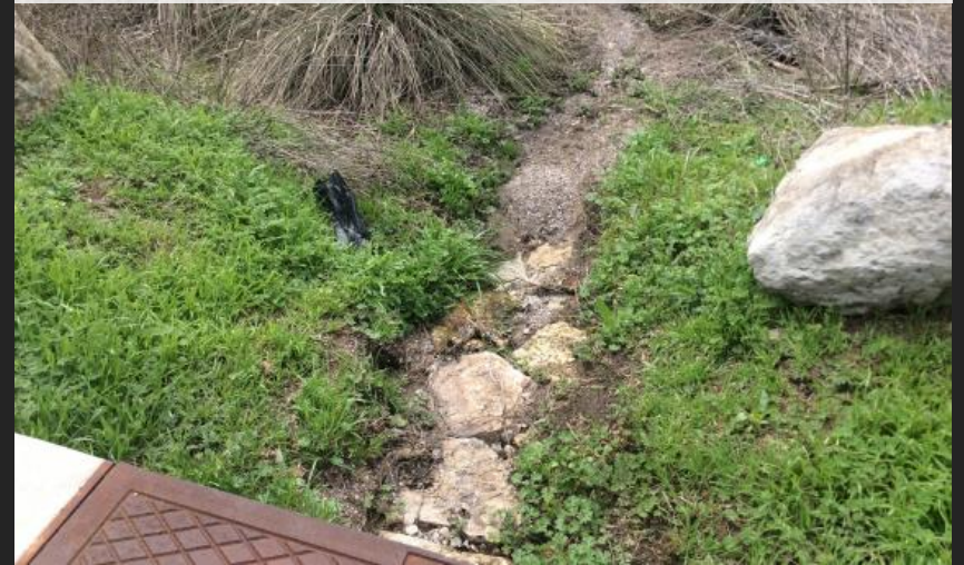
SCOURING AROUND INFLOW
