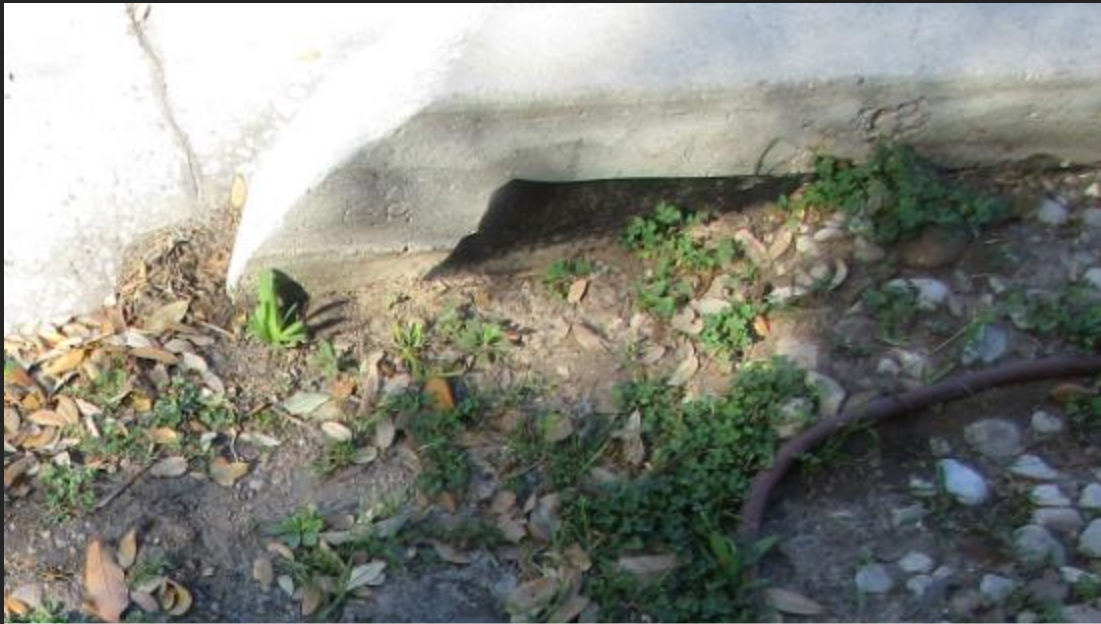
Erosion undercutting concrete curb
