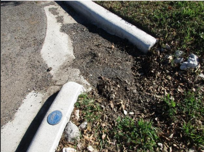
SEDIMENT BLOCKING INFLOW
