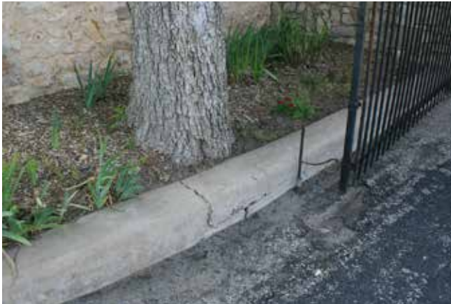
Figure 451. A cracked portion of concrete curb, just inside the entrance gate; the cracking is likely due to pressure from the adjacent pecan tree, which probably is a volunteer, rather than having been planted there. (John Milner Associates)
