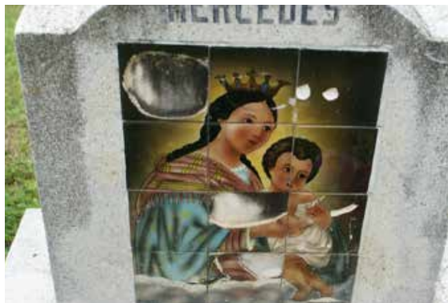
Figure 508. Damage to tile from rocks thrown by mowers (McDoux Preservation, AM-DSC08676)
