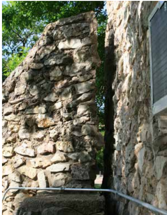
Figure 537. The wall has completely separated from the adjacent building. (John Milner Associates)
