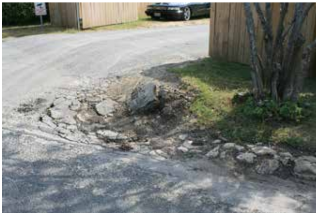
Figure 453. Damage to the road surface from turning vehicles; this has since been repaired (John Milner Associates)
