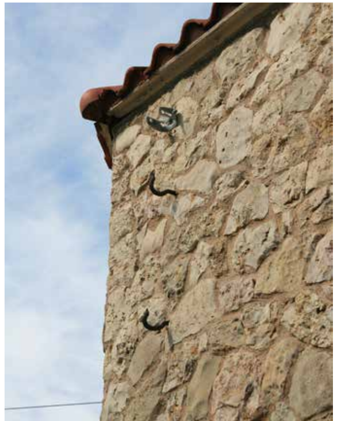
Figure 544. Cable hooks for the former entrance sign are still visible on the exterior of both the tower and the chapel. (John Milner Associates)
