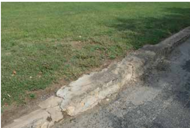
Figure 449. Poor repair of the rock curb lining the entrance drive (John Milner Associates)
