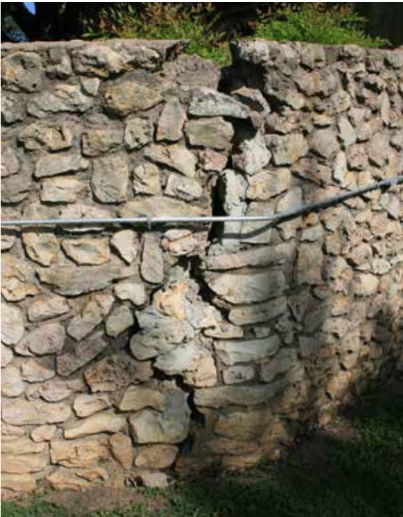
Figure 536. Severely cracked portion of the wall, with attempted repair visible below the steel conduit (John Milner Associates)
